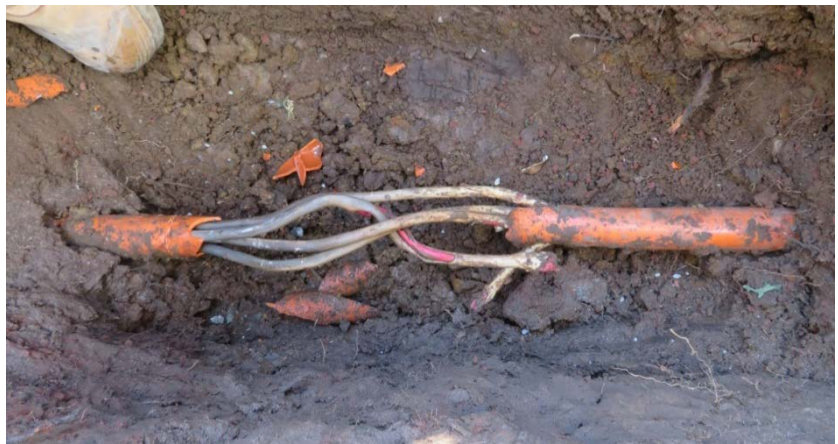
Photo 2: The damaged cable
