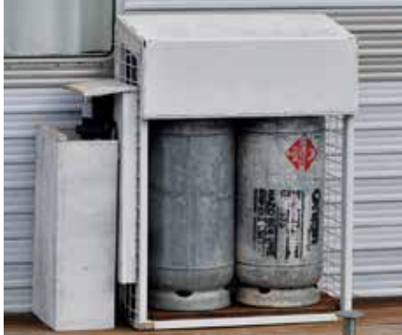
Figure 2, 3 and 4: LPG cylinder compartments and lockers
