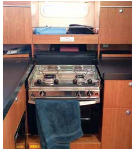
Figure 11: LPG cooker installed on a gimbal
